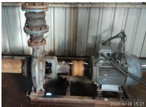
Gambar 2 Pompa Sentrifugal Intake B
